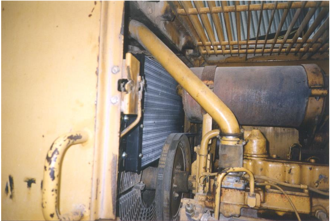
Condenser as viewed from right side.
